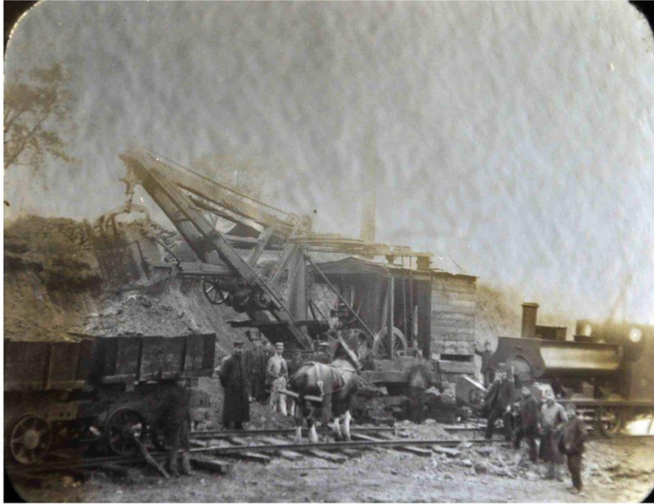
Figure 87. Steam excavator used during Katrine aqueduct construction, 1880s. Note the use of horses and temporary track and steam engine.
