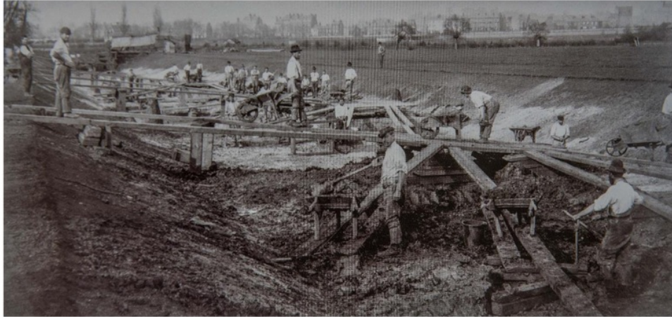
Figure 91. Cherwell New Cut being hand-excavated in 1884. Note extensive use of spades, wheelbarrows and wooden planking. Compare with Figure 84.
