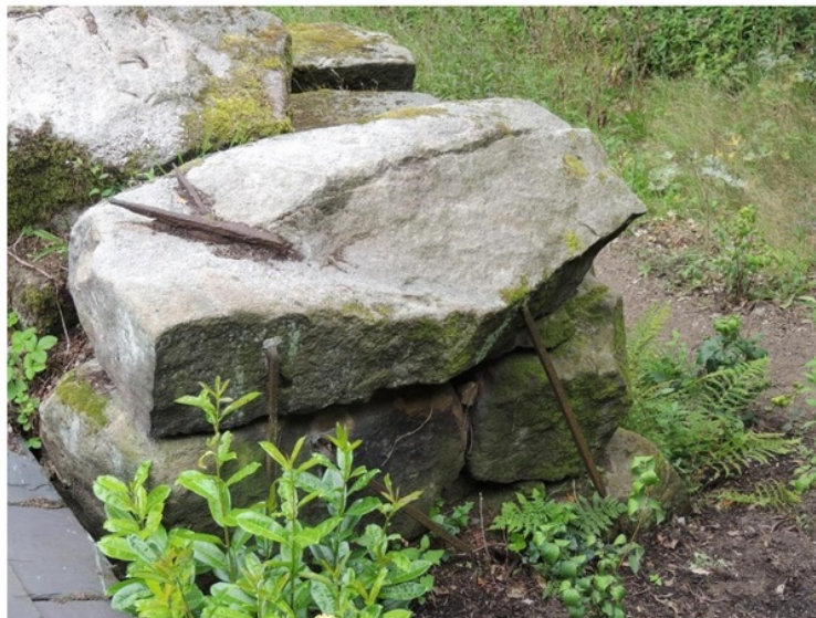
Figure 70. A 19th century metal cramp and remains of ironwork holding rocks together at Chatsworth.
