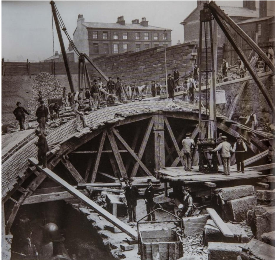
Figure 86. Widening the tunnel at Edge Hill, Liverpool c1872. Note use of hand-cranked derrick cranes, wooden scaffolding and a steam train in bottom left had corner.
