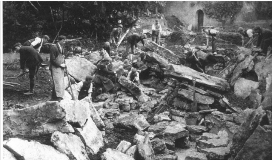
Figure 85. Constructing the ravine at Lilford Hall, Northamptonshire. Note use of shovels, pickaxes and levers.
