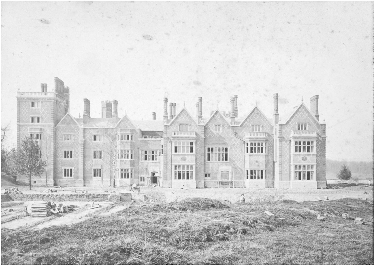
Fig. 123. Building in progress and the start of the terraces, circa 1870s. RIBA 20039/2.
