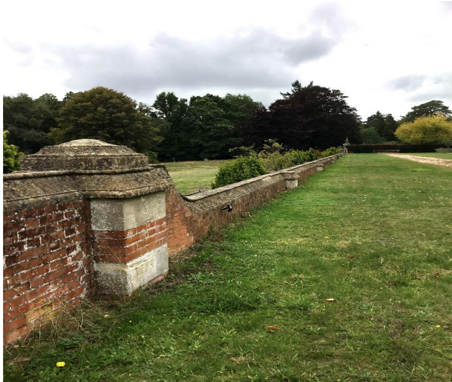
Fig. 207. The terrace wall with piers where the vases and statues would have stood. 2020.
