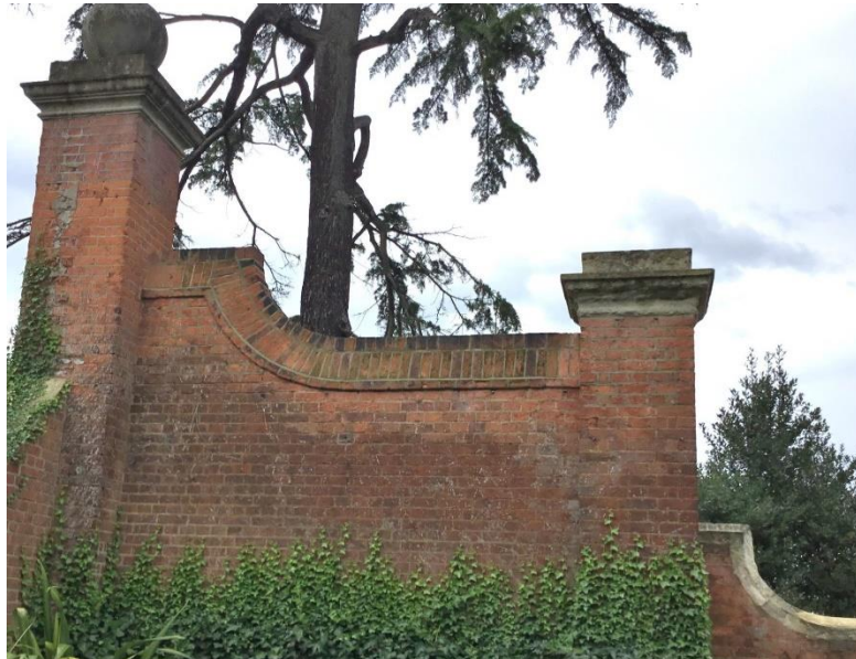
Fig. 189. The brick pier and sloping wall at Warren House in the Devey sketch of 1884. 2019.
